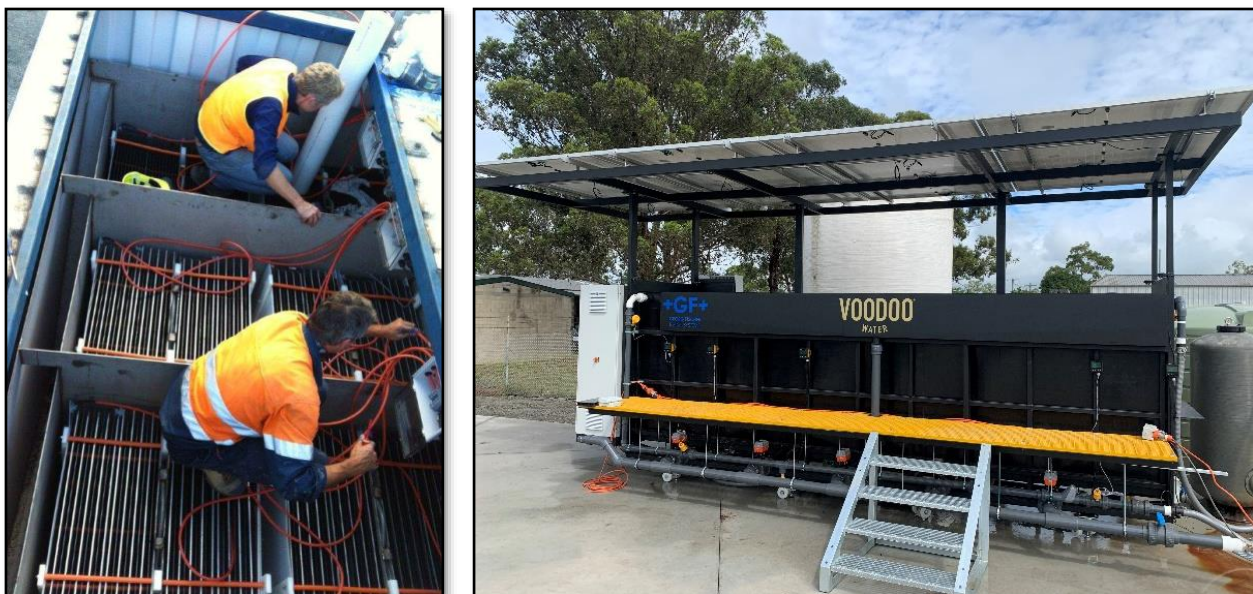
Figure 3 Replacement of reactor plates and elevation view of solar powered electrocoagulation reactor
