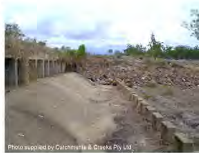
Photo 8 – Note use of impact blocks to stabilise the location of the hydraulic jump
