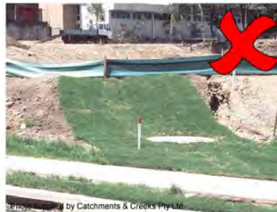
Photo 6 – Turf chute with poorly-defined inlet profile causing flow bypass
