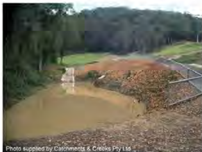
Photo 21 – Sediment basin with poor access for de-silting operations
