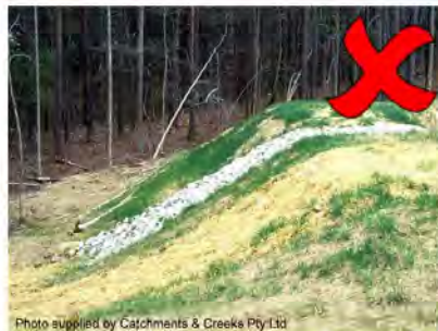
Photo 14 – A suitable energy dissipater must be constructed at the base of the spillway
