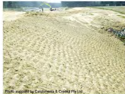
Photo 2 – Corrugated (roughened) surface
