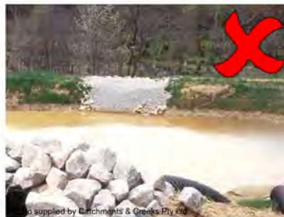
Photo 20 – Spillway crest with inadequate depth or profile
