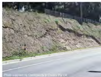
Photo 4 – Slippage of topsoil from steep cut batter
