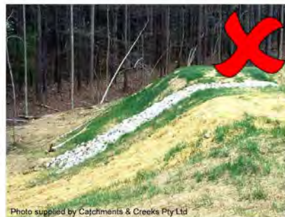
Photo 8 – A suitable energy dissipater must exist at the base of the spillway
