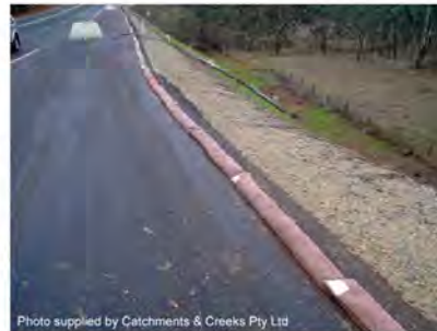
Photo 4 – Sandbag flow diversion berm used to minimise surface flow over a recently seeded embankment
