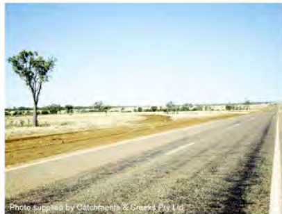
Photo 1 – Diversion drains (centre) collect stormwater from roadside table drains, then releases the water as sheet flow via a level spreader
