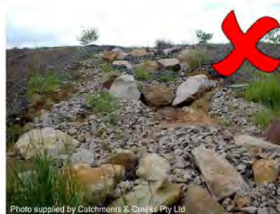
Photo 8 – Erosion caused by inadequate rock size and water bypassing around the poorly located boulders
