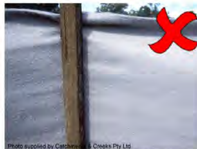
Photo 6 – Filter cloth MUST NOT be used unless used in the construction of a 'Filter Fence' adjacent to a stockpile
