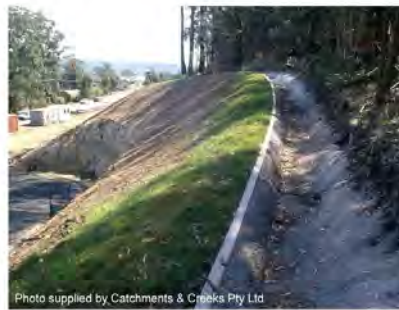
Photo 4 – Permanent catch drain
