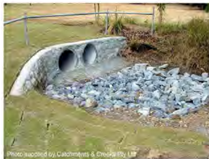
Photo 3 – Rock pad outlet structure
