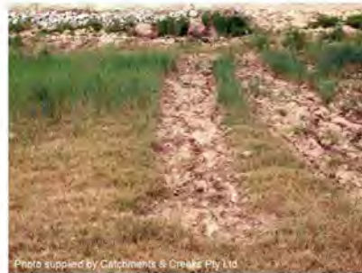
Photo 6 – Rilling down newly vegetated slope cutting through surface roughening
