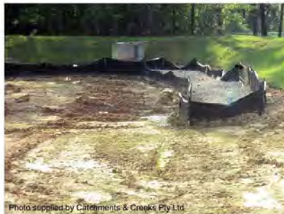
Photo 13 – Low-flow sand filter outlet system on a permanent sediment basin
