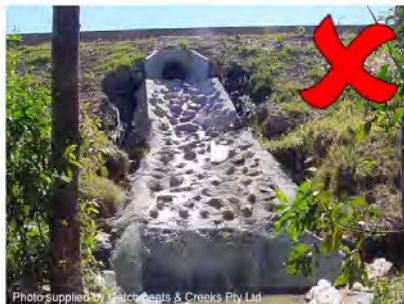
Photo 7 – Severe erosion along edge of chute caused by water spilling out of the chute
