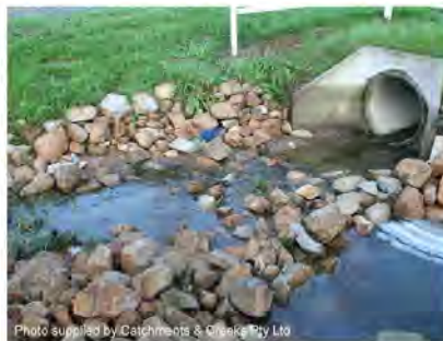
Photo 4 – Rock pad outlet structure
