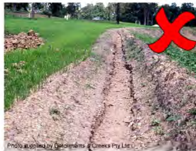
Photo 6 – Velocity-induced bed scour within a catch drain
