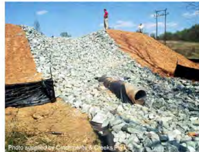
Photo 2 – Rock lined basin spillway and energy dissipater
