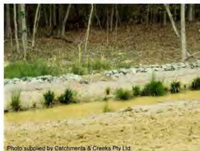
Photo 5 – Sediment trench (with rock filter dam outlet system) located at the base of a fill embankment
