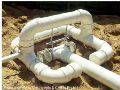
Photo 11 – Skimmer outlet system
