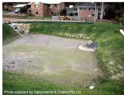
Photo 1 – Type C (dry) sediment basin
