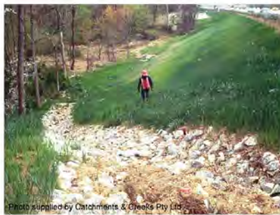
Photo 3 – Rock lined catch drain
