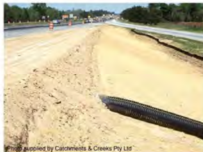
Photo 5 – Earth flow diversion bank used to direct runoff towards the entrance of a Slope Drain
