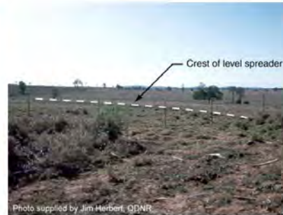
Photo 2 – Level spreader established to discharge stormwater from a diversion drain into the roadside property
