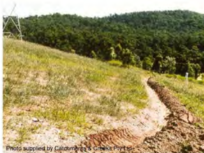
Photo 1 – Unlined catch drain
