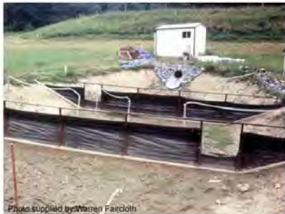
Photo 3 – Inlet chamber can also act as mixing chambers for the addition of flocculants
