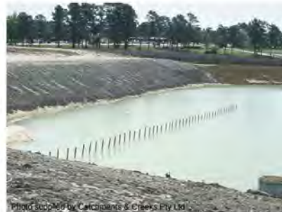
Photo 4 – Internal baffle extending the flow path between the basin inlet (left) and the basin outlet (right)
