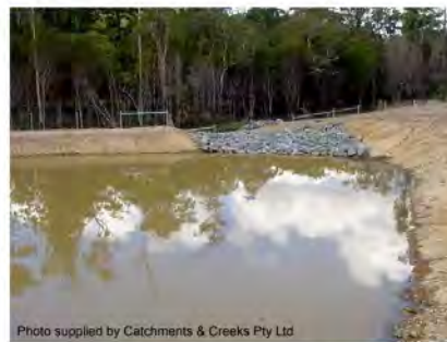
Photo 2 – Type F (wet) sediment basin
