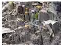
Photo 3 – Raindrop impact erosion
