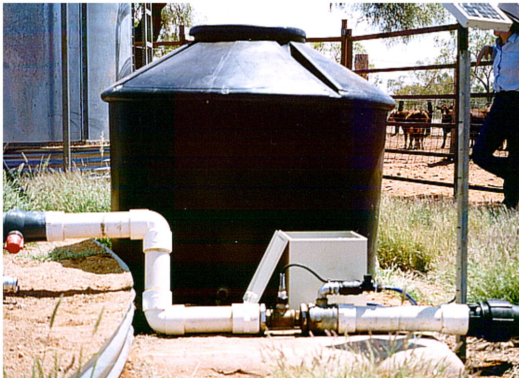
Figure 1. Water medication unit - on property installation
